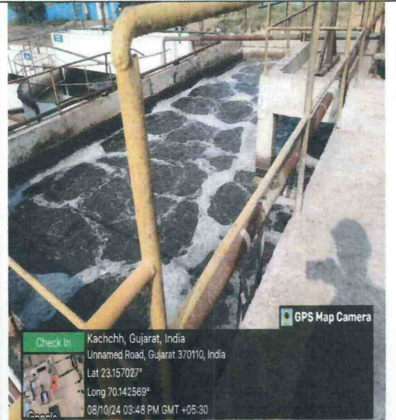
Photograph : 4 Aeration Tank of ETP
